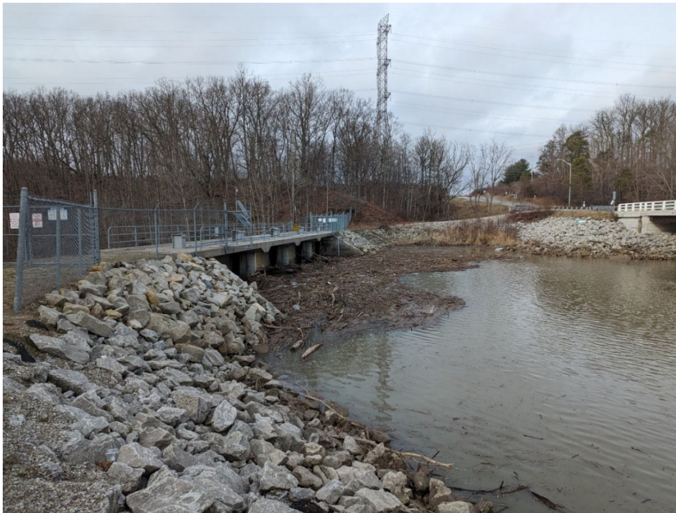
Woody debris accumulated on the upstream face of the Dalewood Dam in January 2024.
