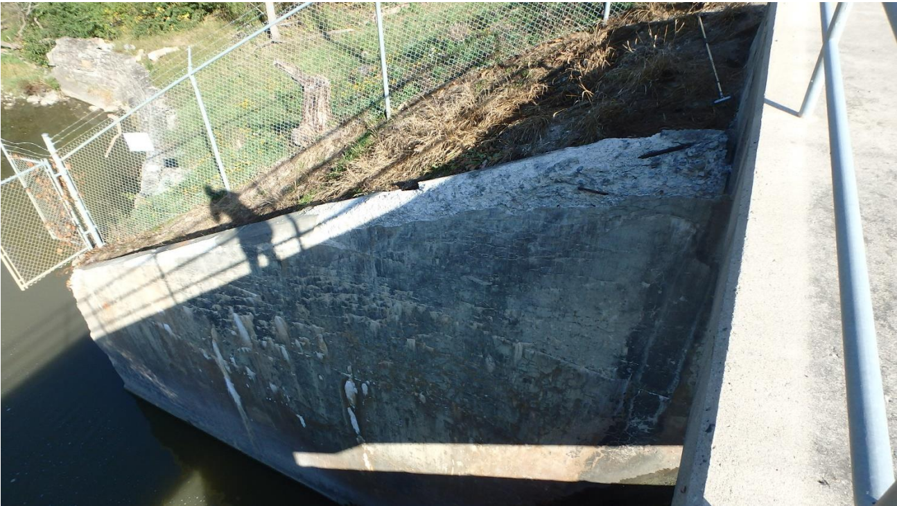
2. Spalling on North Downstream Wingwall
