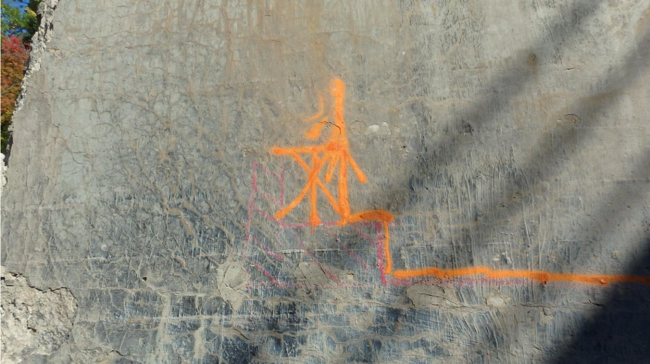
1. Delaminated Area of North Downstream Wingwall
