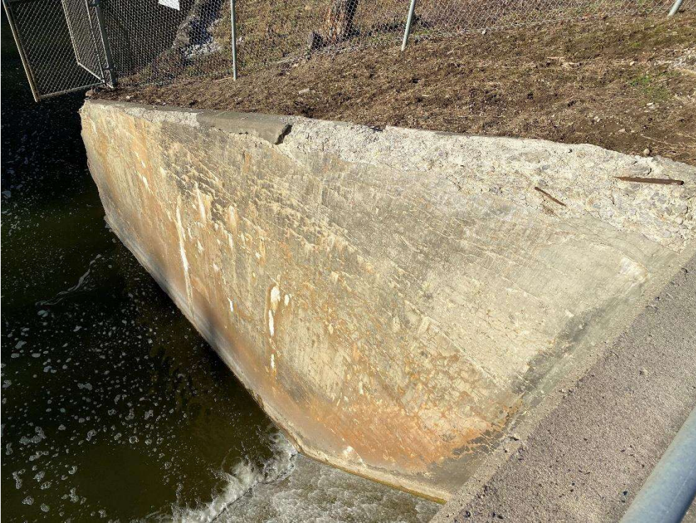
3. Spalling on North Downstream Wingwall – December 14 th , 2022 Inspection
