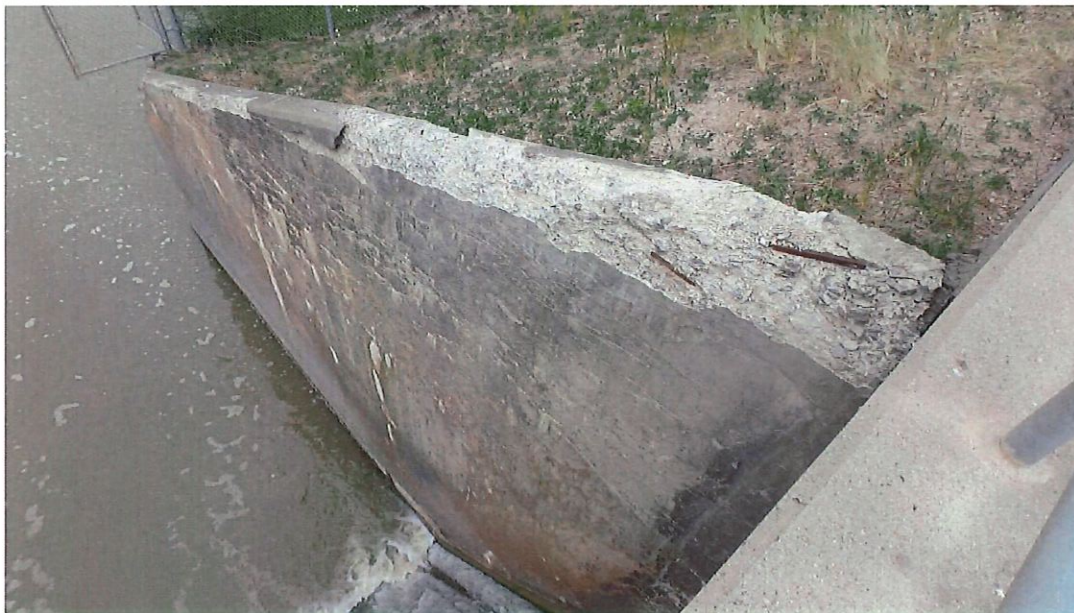
2. Spalling on North Downstream Wingwall
