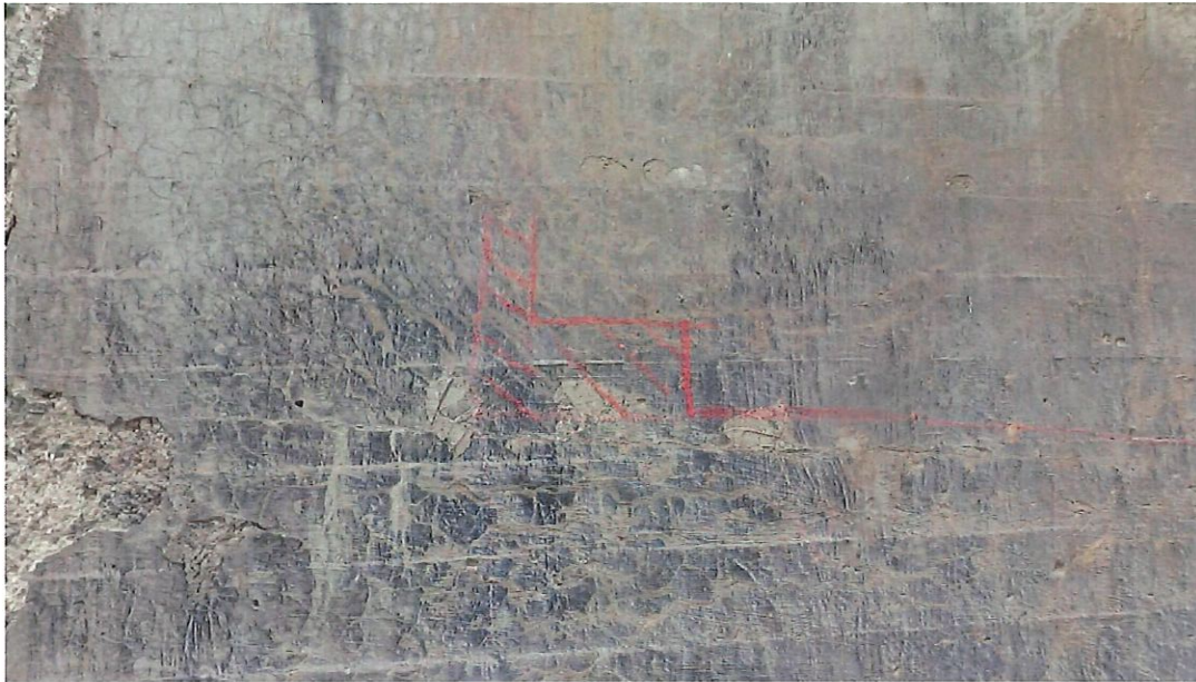
1. Delaminated Area of North Downstream Wingwall
