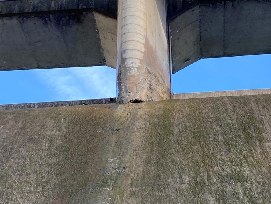
4. Deterioration and Void at Pier
