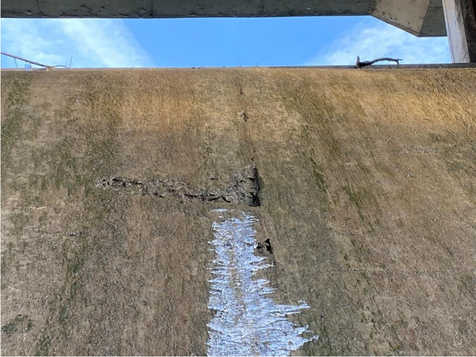
2. Spalling in Spillway Face
