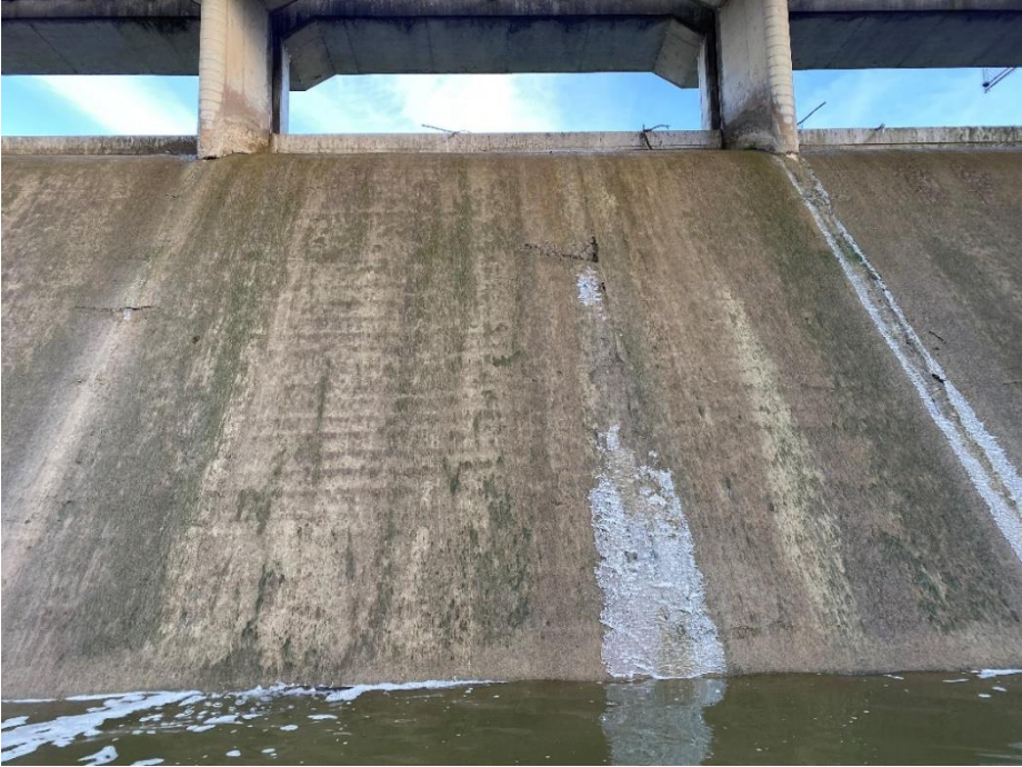
3. Vertical Crack/Construction Joint in Dam Spillway
